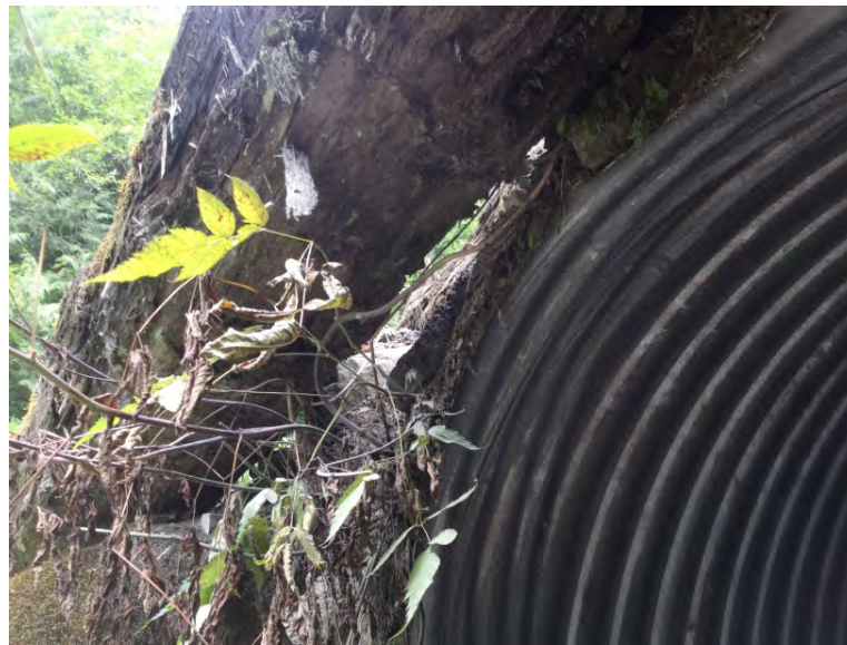
Eroding fill inlet
